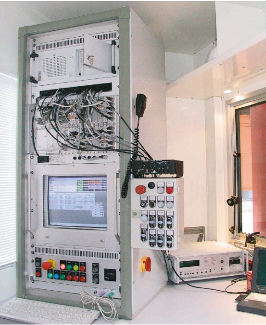
Fig. 7, left: 19" rack with PC, monitor and controller for load application and vehicle hydraulics, together with UPM100 multipoint measurement amplifier from HBM
