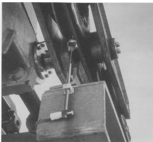
Fig. 7: At bottom station, track-cable entry angle is measured with inductive displacement transducer
