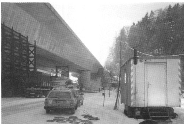
Fig. 4: The measurement station set up in a builder's trailer on the left bank of the river; the auxiliary supports for the girder can be seen in the left of the picture
