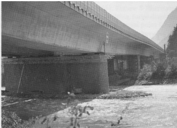
Fig. 2: View of the bridge and river pier from the downstream side after initial safety work had been carried out
