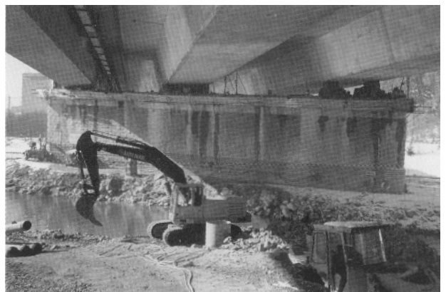
Fig. 3: View of the river pier from the right-hand bank after lifting the girders, showing the temporary prefabricated bearing stacks
