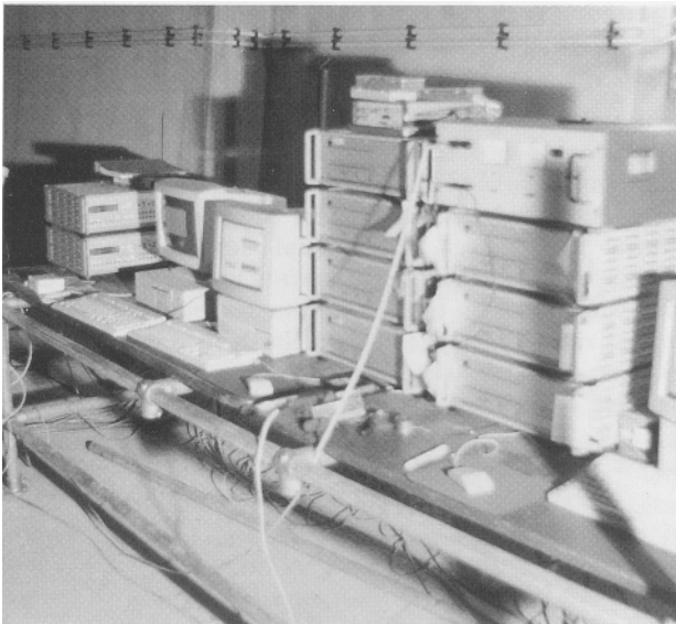
Fig. 5: View of the measurement system installed inside the bridge girder box.
