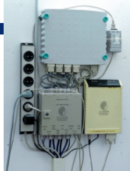
Figure 7: Instrumentation in the measuring room
