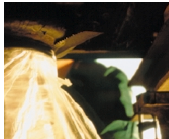
Fig. 11: Making a saw cut between the upper end of the column and the capital; a plastic sheet protects the measuring points during work at the top of the column
