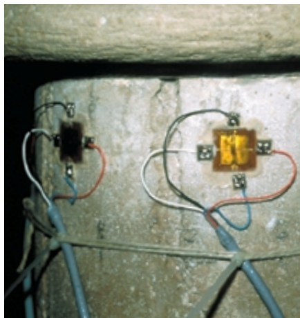
Fig. 8a: Measuring points on the upper edge of the column before masking, cord being used to relieve strain on cable connections
