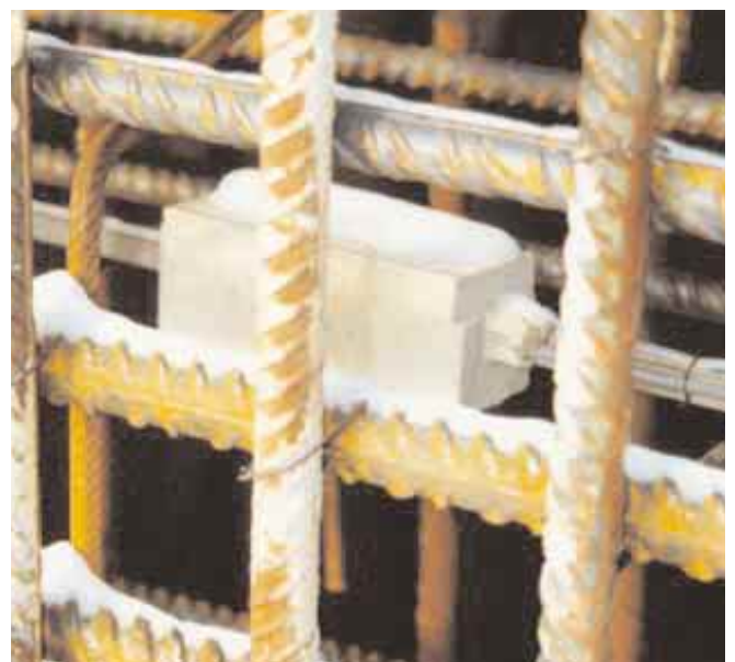
Fig. 11: Measurement transducer integrated into the reinforcement
