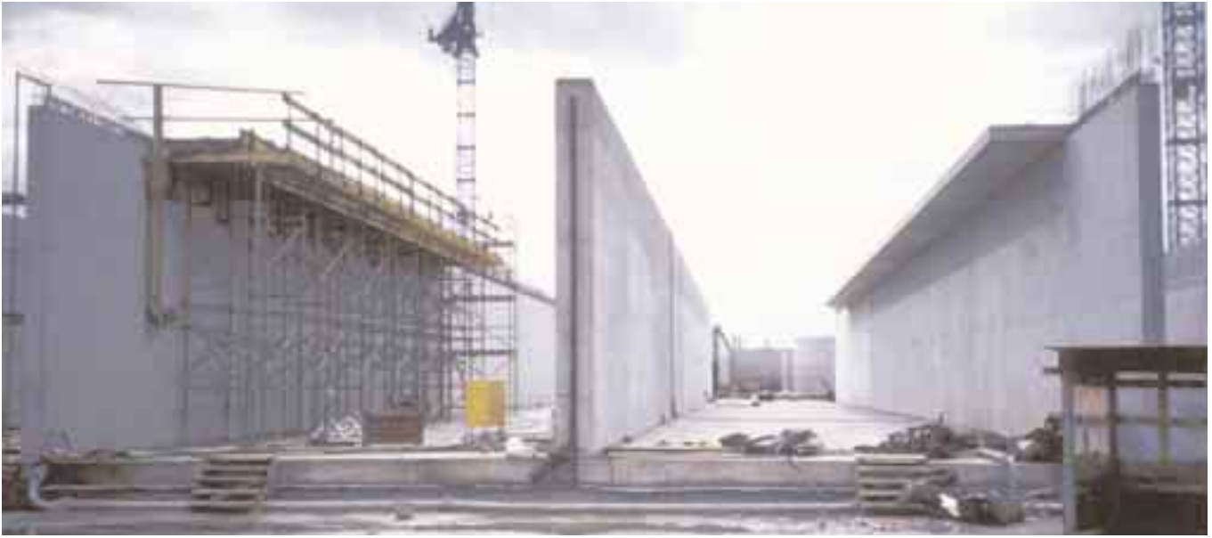
Fig. 8: Site of the Wassmannsdorf clarification plant near Berlin
