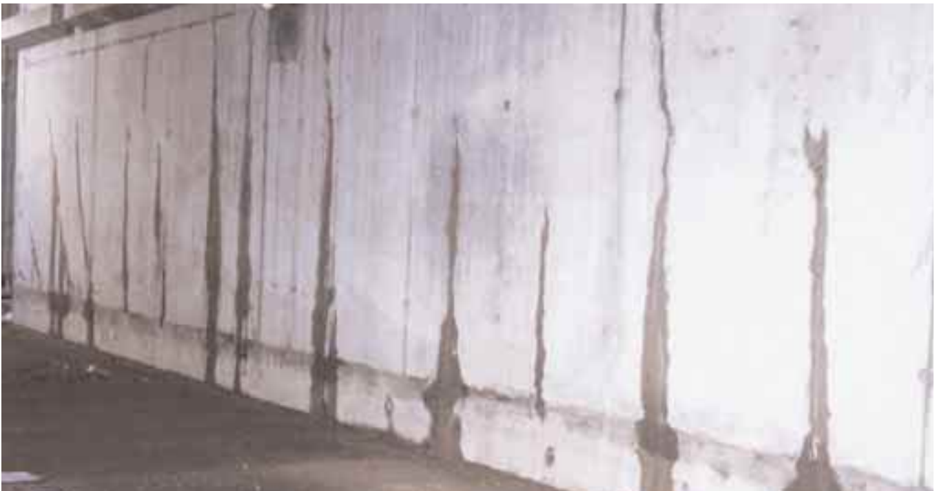
Fig. 1: Hydration cracks in a settling basin during fill test
