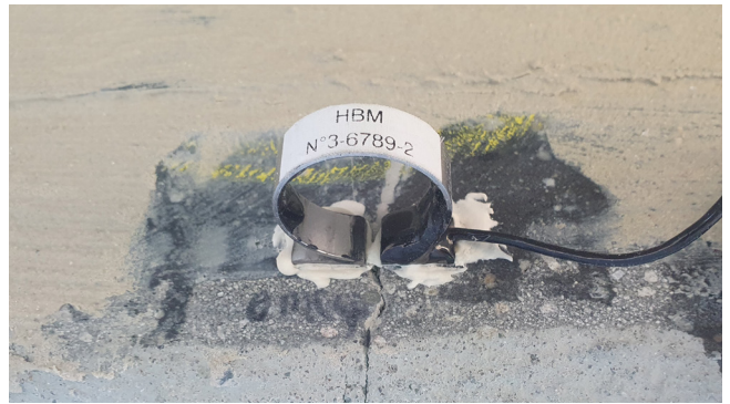
Figure 5: Omega sensor installed at existing site of crack
