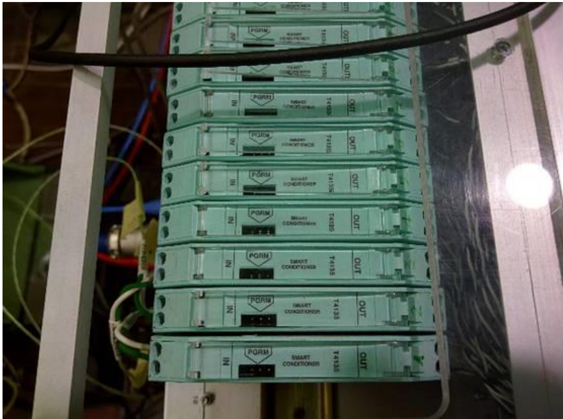
Fig. 4.a: Programmable isolation amplifiers for temperature measurement
