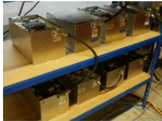
Fig. 5: Lithium battery bank to supply the inverter
