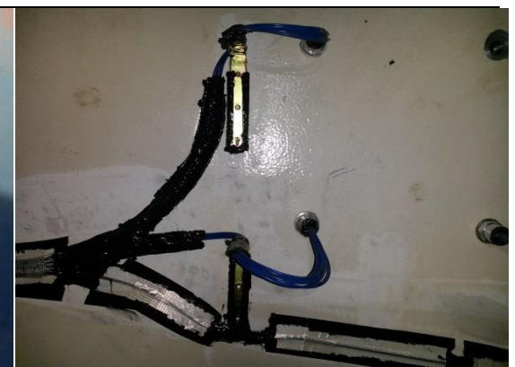
Fig. 26: Flanges (seen from the inside of the pipe)
