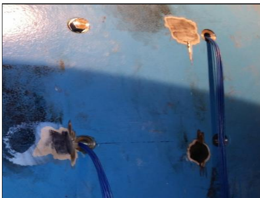
Fig. 25: Cable egress (seen from the outside of the pipe)
