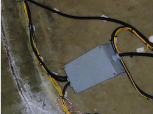
Fig. 2.12 Protection boxes for extra cable and connections
