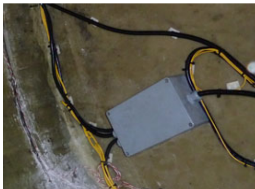
Fig. 2.4 Protection boxes for extra cable and connections
