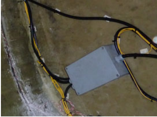
Fig. 2.9 Protection boxes for extra cable and connections
