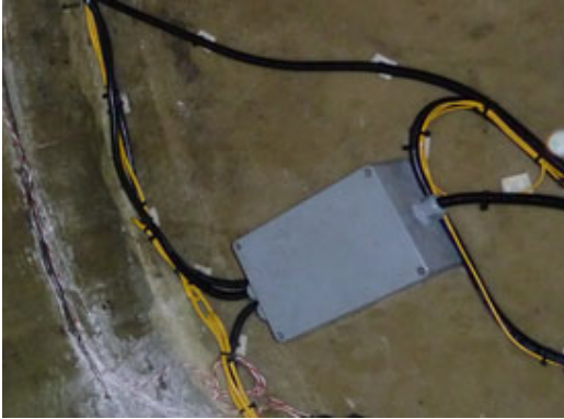
Fig. 2.26 Protection boxes for extra cable and connections
