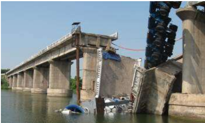
Fig.1: Bridge Collapse (in pixabay.com/de - public domain)
