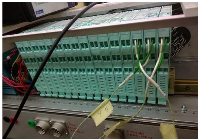
Fig. 4.b: Programmable isolation amplifiers for temperature measurement
