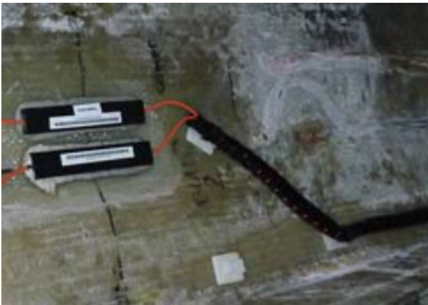
Fig. 2.30 Cable protected with corrugated tubes
