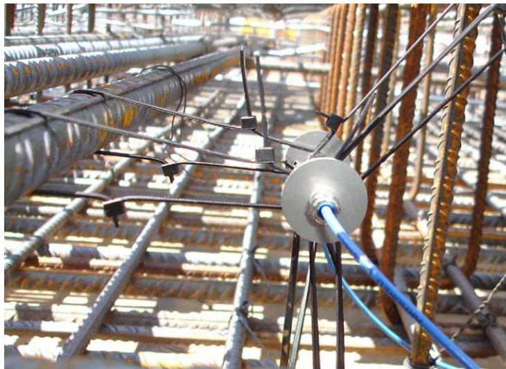
Figure 4. Embedded strain sensor being installed on a bridge's deck before the concrete is poured.
